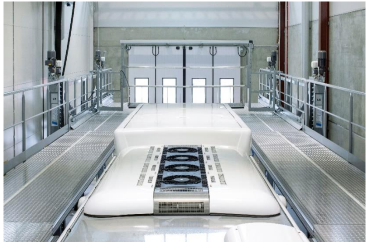
Roof working platforms for electrical buses
